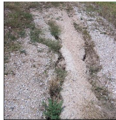
Storm water erosion gullies and rills
