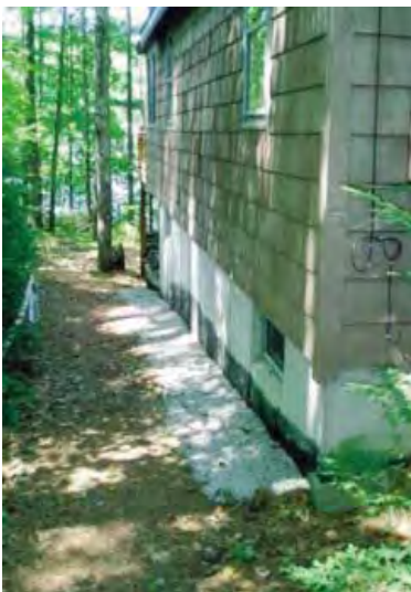
An infiltration trench was constructed to catch roof runoff at this lakeside home.
