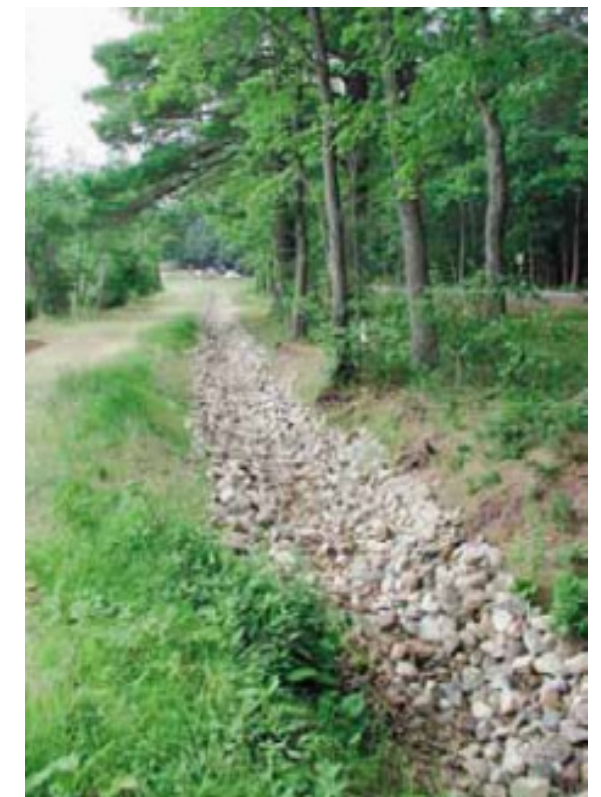
A swale constructed along this roadway captures road runoff and prevents it from entering the lake, to the left.
